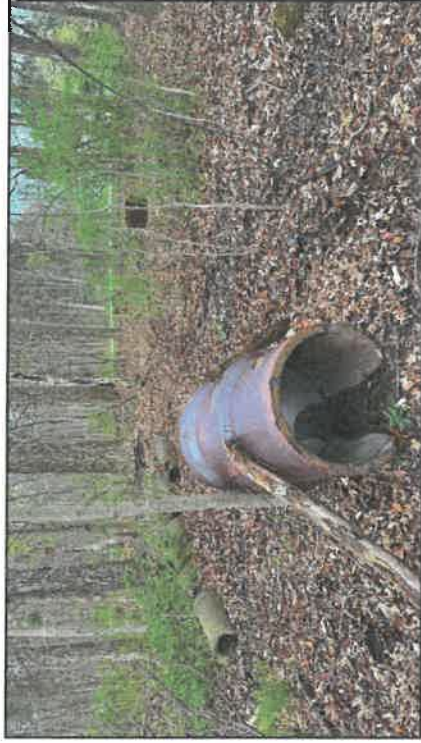
4. Looking north at a number of tile and cement culverts located in the eastern forest across from the Village Hall.
